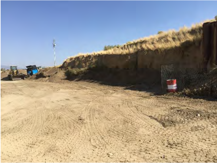
Photo #4: Materials stockpiled against the highwall on the south side of the LMO boundary. The stockpiled material has decreased in volume. Photo taken September 24, 2020.
