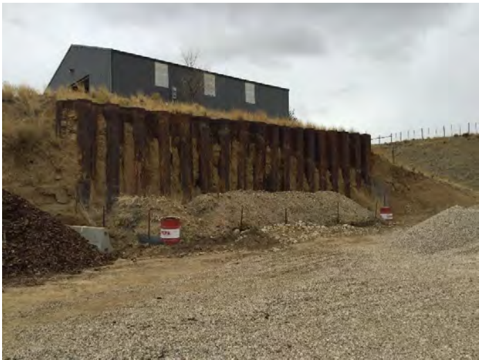
Photo #10: QLN installed and maintains a fence around the perimeter of the steel retaining wall. Mining outside the LMO boundary has resulted in material damage to the steel retaining wall.
