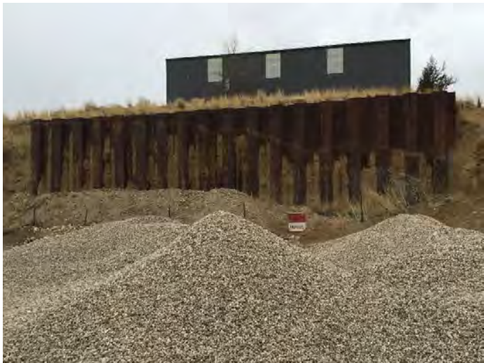
Photo #9: QLN installed and maintains a fence around the perimeter of the steel retaining wall. Mining outside the LMO boundary has resulted in material damage to the steel retaining wall.
