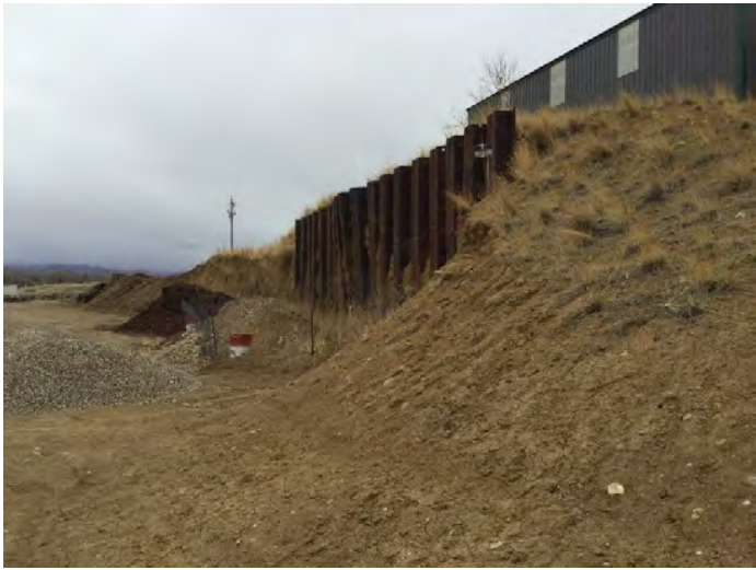
Photo #8: General overview of steel retaining wall looking east. Mining has resulted in material damage to the steel retaining wall. The middle of the wall is slowly bulging out towards the north.
