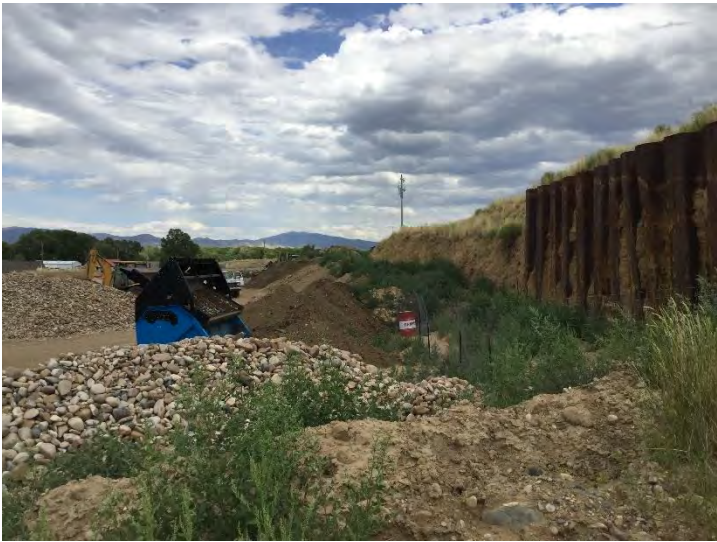
Photo #2: Materials stockpiled against the highwall on the south side of the LMO boundary. Photo taken July 14, 2020.
