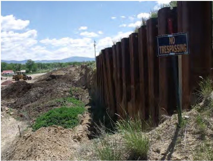
Photo #1: General overview of mining towards steel retaining wall looking east. Mining has occurred outside the LMO legal description.
