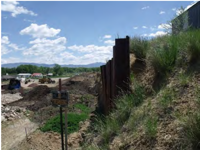
Photo #7: General overview of steel retaining wall looking east. Mining has resulted in material damage to the steel retaining wall. The middle of the wall is slowly moving out towards the north.
