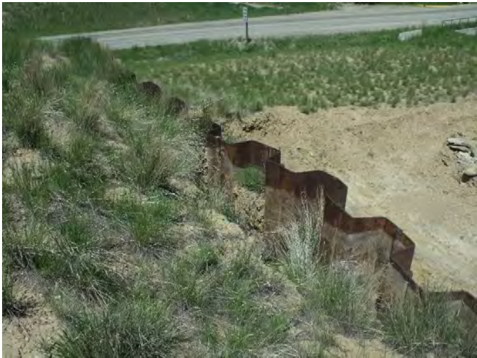
Photo #8: General overview of steel retaining wall. Water is piping behind the retaining wall causing material damage.
