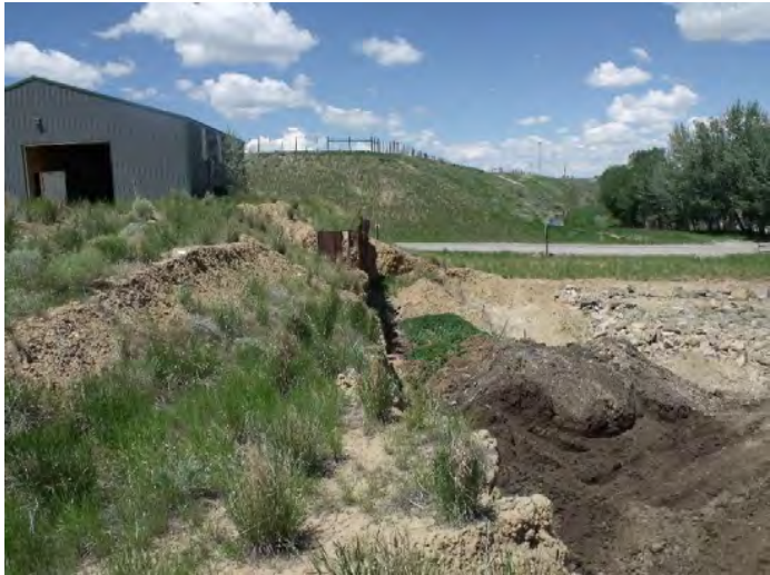
Photo #5: General overview of the top of the steel retaining wall and LMO legal description. Mining has occurred outside the LMO legal description.
