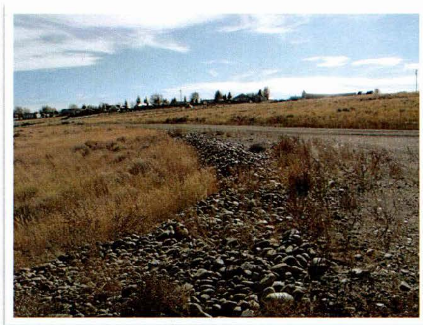
Photo #6: Road, fill material, and sediment control structure constructed at the 10 acre tract of land.
