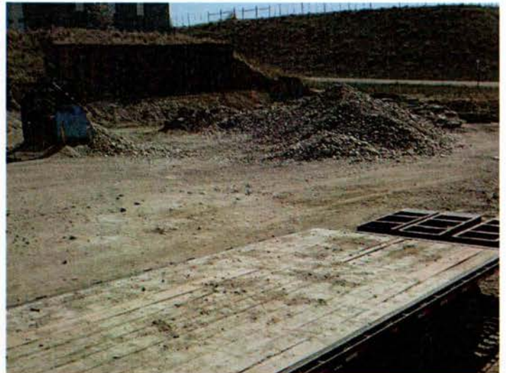
Photo #15: June 12, 2018 - LMO 1496ET general overview of the site and alluvium stockpile.
