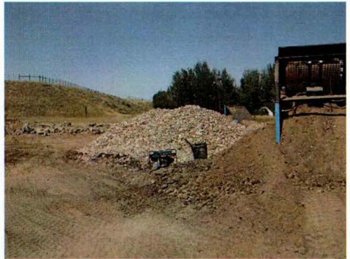
Photo #19: August 29, 2019 - LMO 1496ET general overview of the site and alluvium stockpile.
