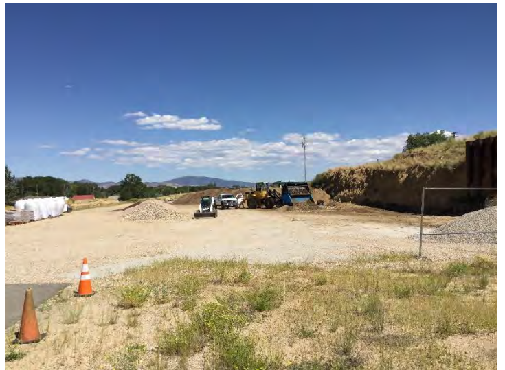
Photo #8: General overview of steel retaining wall looking east. Mining has resulted in material damage to the steel retaining wall. The middle of the wall is slowly bulging out towards the north. Photo taken August 8, 2022.
