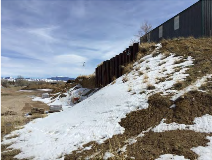
Photo #1: General overview of steel retaining wall looking east. Mining has resulted in material damage to the steel retaining wall. The middle of the wall is slowly bulging out towards the north. Photo taken March 15, 2022.
