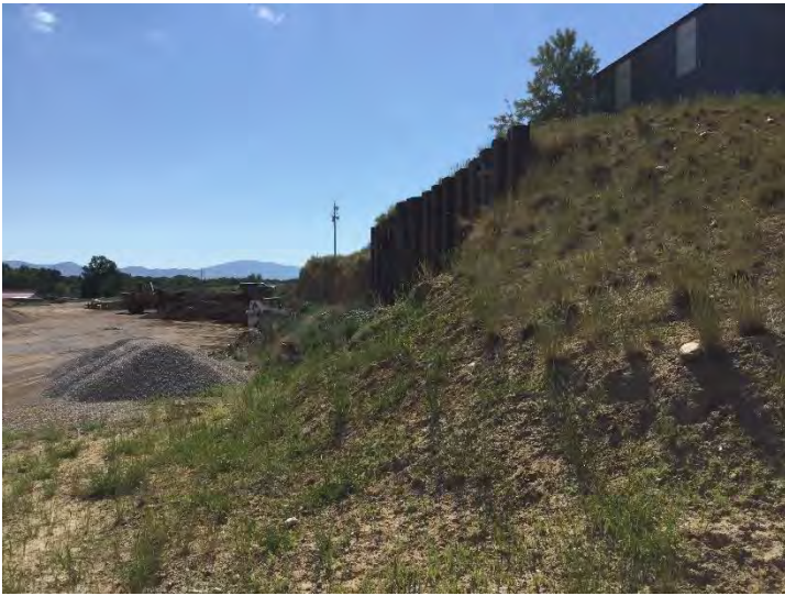
Photo #5: General overview of steel retaining wall looking east. Mining has resulted in material damage to the steel retaining wall. The middle of the wall is slowly bulging out towards the north. Photo taken July 12, 2022.
