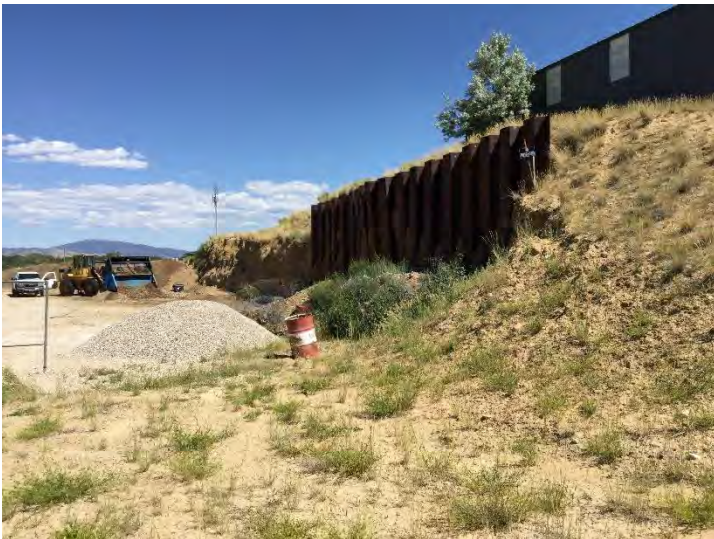
Photo #7: General overview of steel retaining wall looking east. Mining has resulted in material damage to the steel retaining wall. The middle of the wall is slowly bulging out towards the north. Photo taken August 8, 2022.
