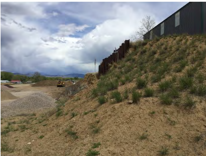
Photo #3: General overview of steel retaining wall looking east. Mining has resulted in material damage to the steel retaining wall. The middle of the wall is slowly bulging out towards the north. Photo taken June 3, 2022.
