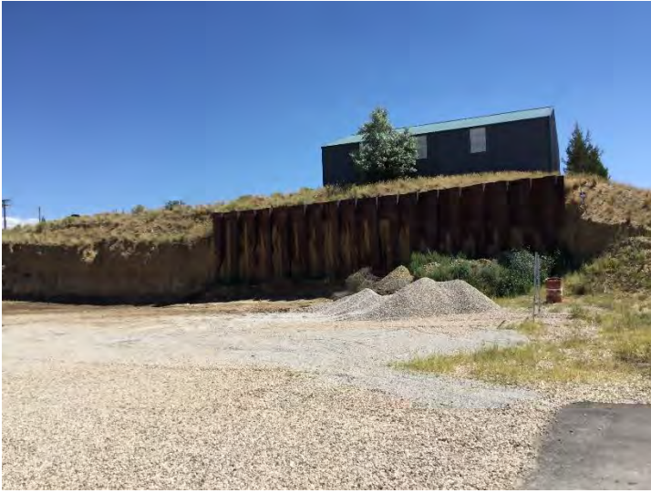
Photo #9: Quality Landscape has removed the fence, berm, and signage from sheet pile retention wall area. Quality Landscape must reinstall the fence, berm, and signage. Photo taken August 8, 2022.
