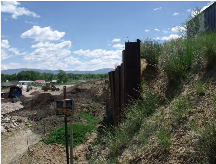
Photo #7: General overview of steel retaining wall looking east. Mining has resulted in material damage to the steel retaining wall. The middle of the wall is slowly moving out towards the north.
