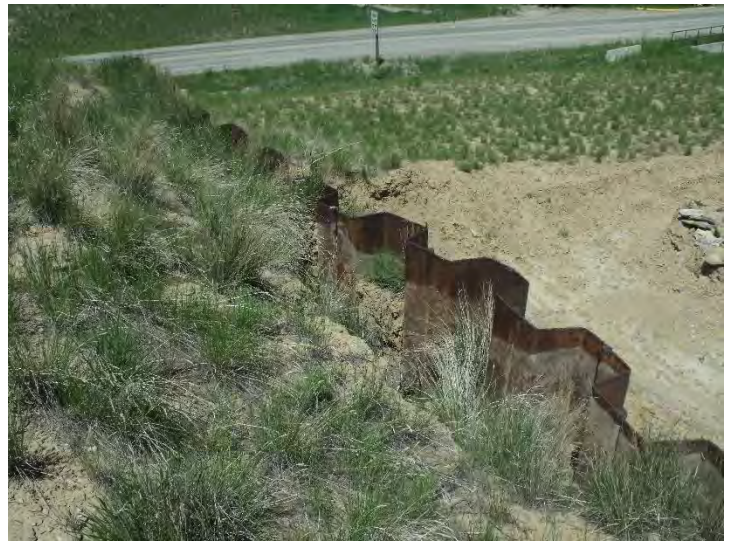
Photo #8: General overview of steel retaining wall. Water is piping behind the retaining wall causing material damage.
