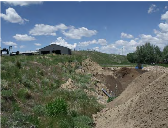
Photo #3: General overview of southern LMO boundary looking west. Survey stakes marking Lots 1 thru 11. Mining has occurred outside the LMO legal description.
