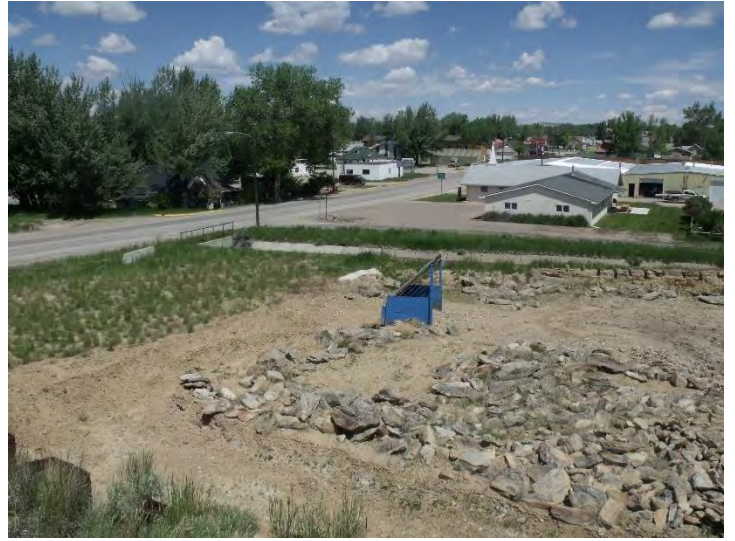
Photo #6: General overview of sump. The small sump is functioning appropriately.
