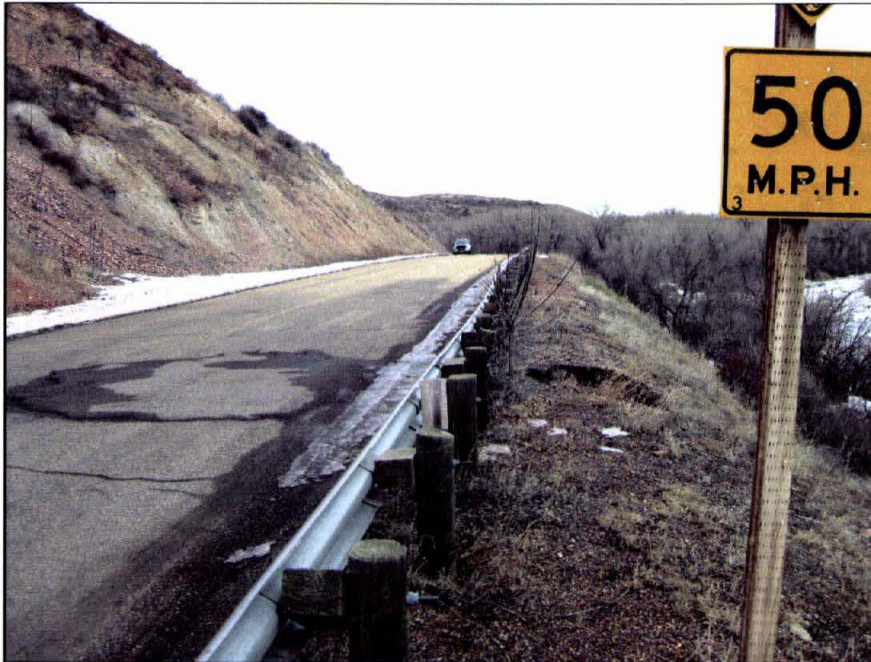
Photo 1. Looking east down the Acme Road (County Road 345). Note asphalt patch where subsidence has occurred under the road in the past. Note active subsidence pit immediately right of the guardrail.
