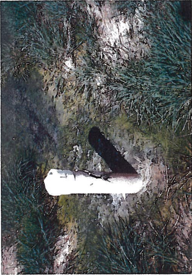
w.w. spilling out of riser pipe
