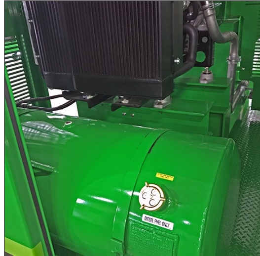
Fuel Tank - Open Side Door
