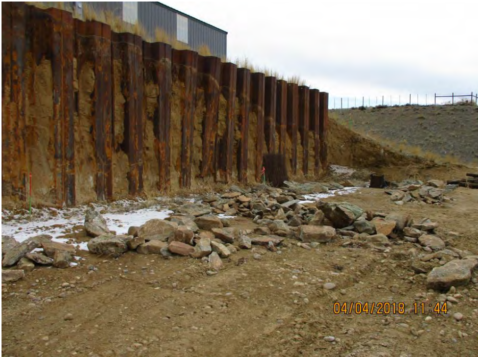
Picture taken by State Mine Inspector 4/4/2018
