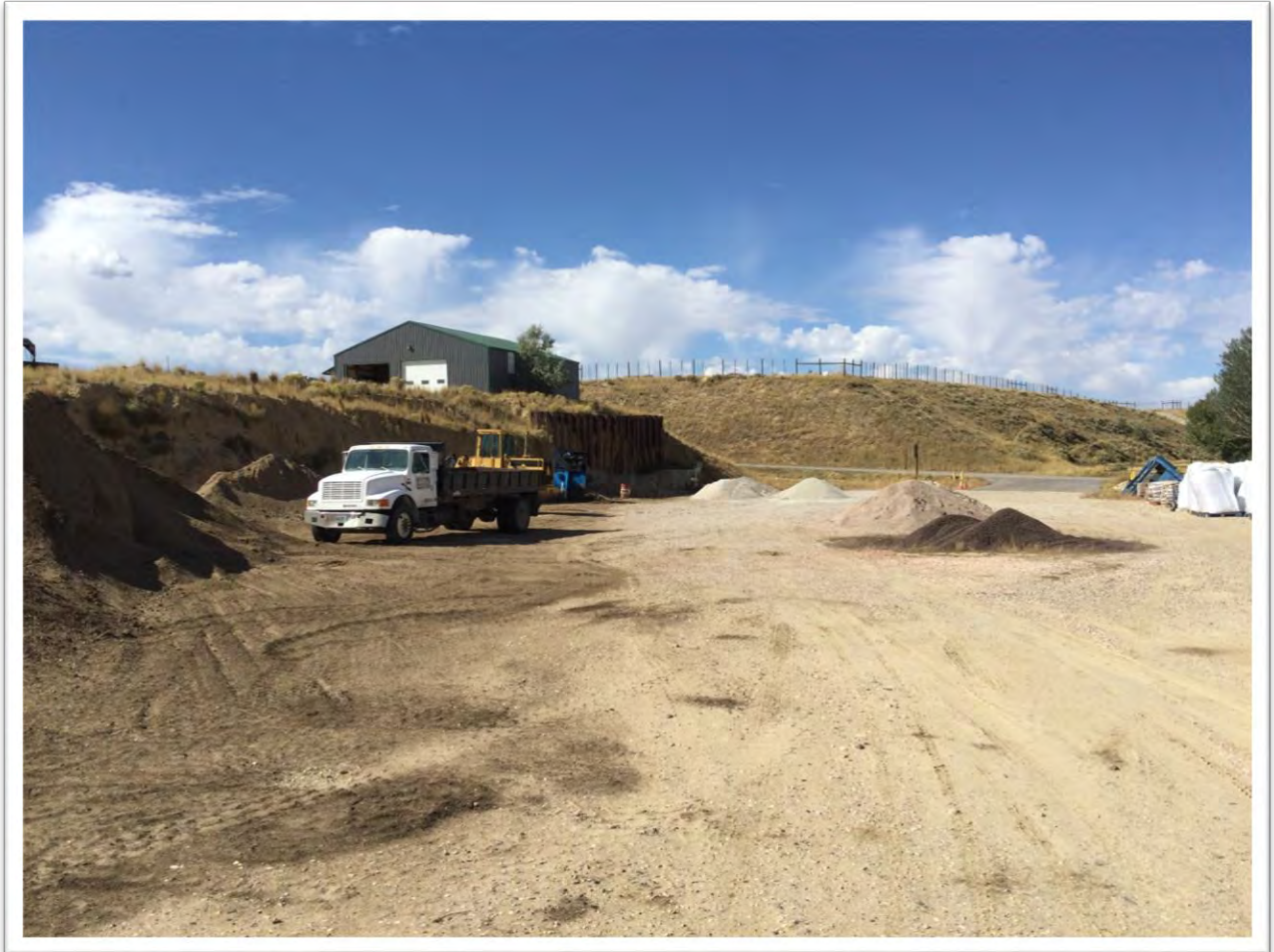
Photo #1: Quality Landscape reinstated the fencing and warning signs around the sheet pile wall.
