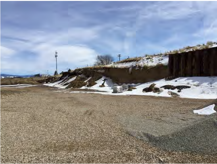
Photo #2: General overview of the LMO. Materials stockpiled against the highwall on the south side of the LMO boundary. Photo taken March 15, 2022.
