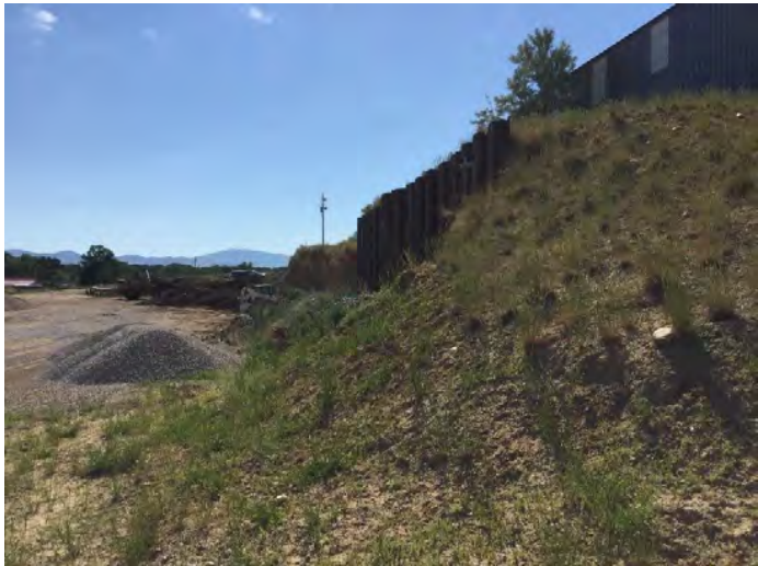
Photo #5: General overview of steel retaining wall looking east. Mining has resulted in material damage to the steel retaining wall. The middle of the wall is slowly bulging out towards the north. Photo taken July 12, 2022.
