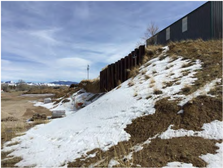
Photo #1: General overview of steel retaining wall looking east. Mining has resulted in material damage to the steel retaining wall. The middle of the wall is slowly bulging out towards the north. Photo taken March 15, 2022.
