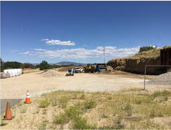
Photo #4: General overview of the LMO. Materials stockpiled against the highwall on the south side of the LMO boundary. Photo taken June 3, 2022.
