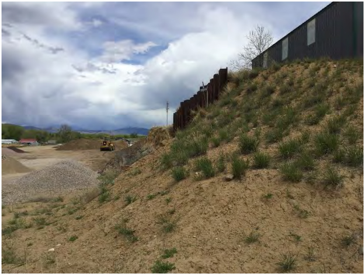
Photo #3: General overview of steel retaining wall looking east. Mining has resulted in material damage to the steel retaining wall. The middle of the wall is slowly bulging out towards the north. Photo taken June 3, 2022.
