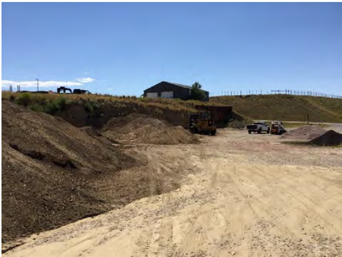
Photo #10: Quality Landscape has removed the fence, berm, and signage from sheet pile retention wall area. Quality Landscape must reinstall the fence, berm, and signage. Photo taken August 8, 2022.
