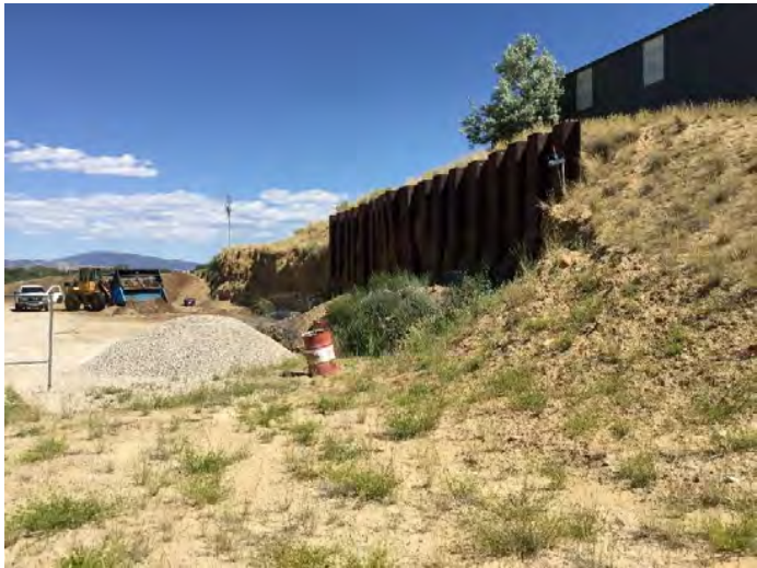
Photo #7: General overview of steel retaining wall looking east. Mining has resulted in material damage to the steel retaining wall. The middle of the wall is slowly bulging out towards the north. Photo taken August 8, 2022.
