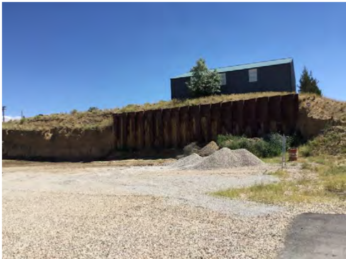
Photo #9: Quality Landscape has removed the fence, berm, and signage from sheet pile retention wall area. Quality Landscape must reinstall the fence, berm, and signage. Photo taken August 8, 2022.
