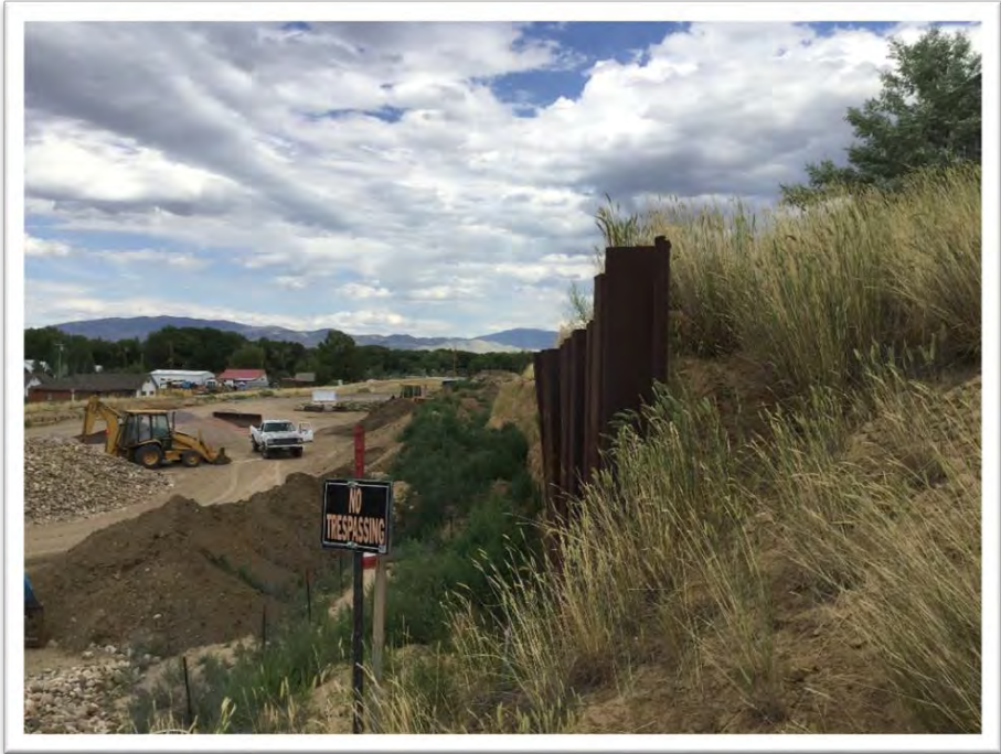
Photo #8: Mining has occurred outside the legal description and has resulted in material damage to steel retaining wall and adjacent property. Photo taken on July 14, 2020.
