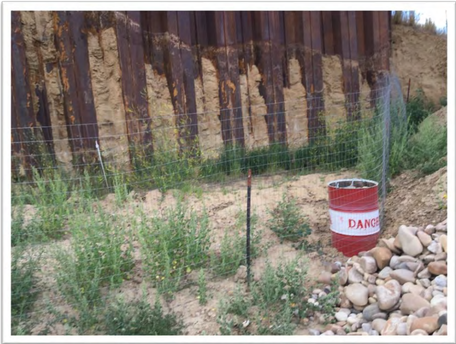
Photo #10: QLN installed and maintains a fence around the perimeter of the steel retaining wall. Photo taken on July 14, 2020.
