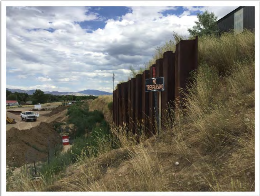
Photo #2: Materials stockpiled against the highwall on the south side of the permit boundary. Photo taken on July 14, 2020.
