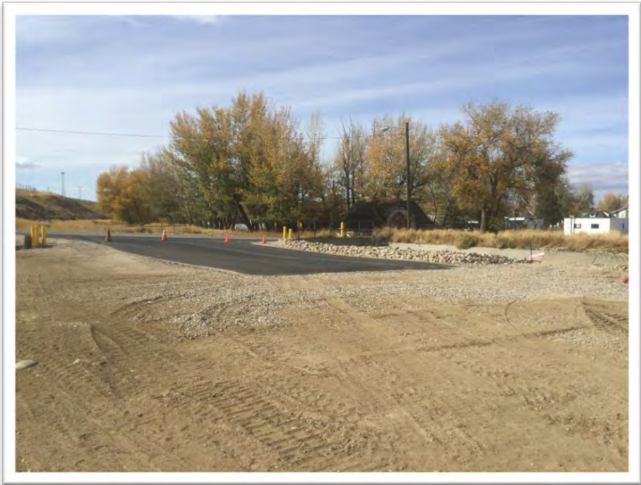
Photo #7: QLN constructed commercial access to the LMO. Photo taken on October 15, 2020.
