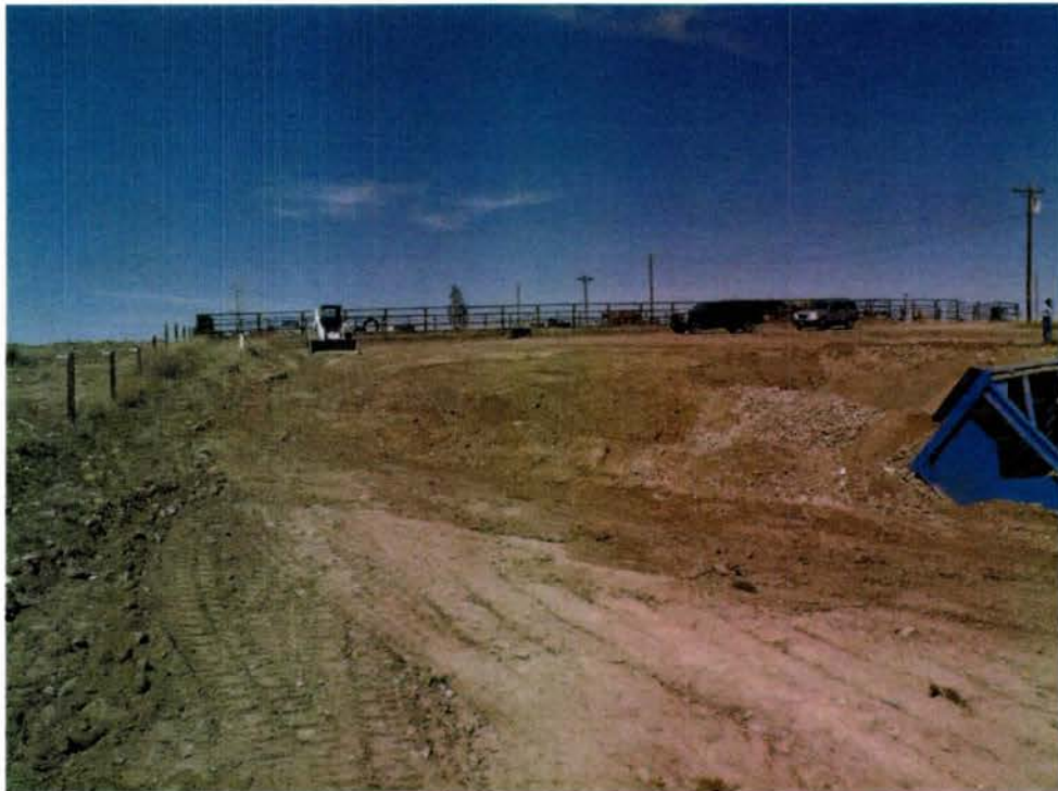
Photo #6: General overview of the property looking west. Mr. Stevens continues to screen the soil from the river cobble. Notice the stockpiles of river cobble has been removed from the property (04/29/2020).
