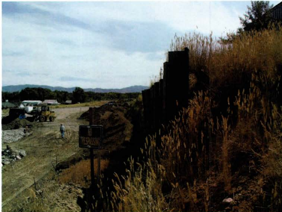
Photo #12: Baseline photograph of the material stockpiles located on the southern side of LMO 1496ET (08/29/2019).
