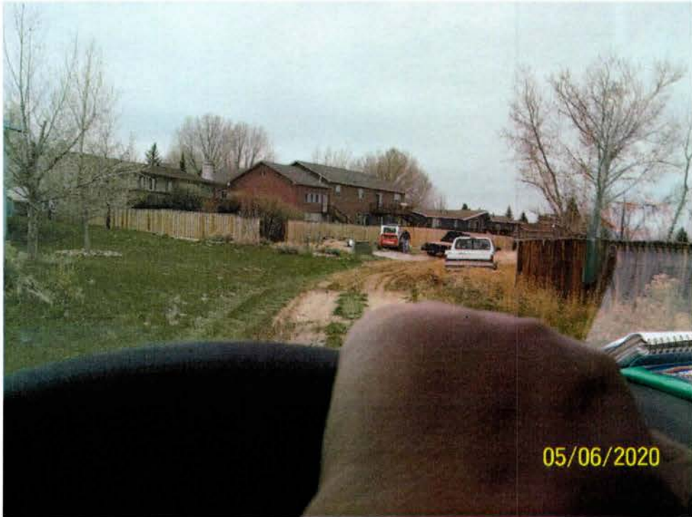
Photo #21: Mr. Stevens working at a private property located at 112 Elk Street. A load of road base has been applied to the alley surface. Mr. Stevens is beside the bobcat walking toward the LQD inspector.
