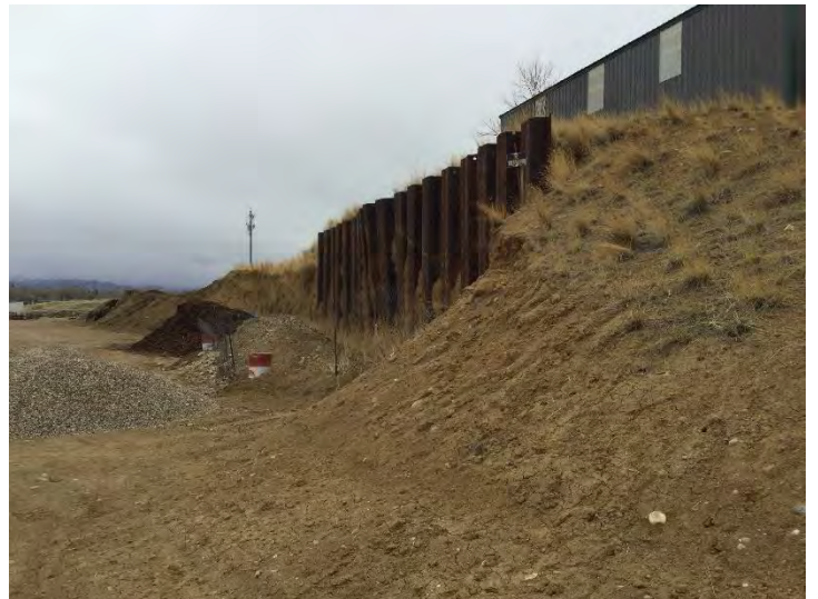
Photo #8: General overview of steel retaining wall looking east. Mining has resulted in material damage to the steel retaining wall. The middle of the wall is slowly bulging out towards the north.
