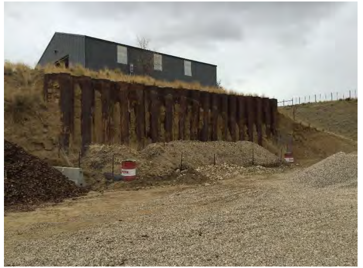
Photo #10: QLN installed and maintains a fence around the perimeter of the steel retaining wall. Mining outside the LMO boundary has resulted in material damage to the steel retaining wall.
