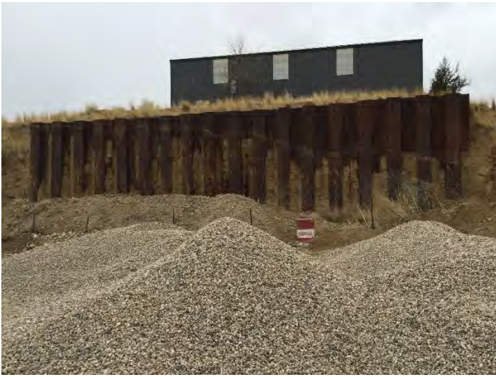
Photo #9: QLN installed and maintains a fence around the perimeter of the steel retaining wall. Mining outside the LMO boundary has resulted in material damage to the steel retaining wall.
