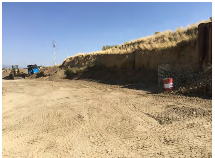
Photo #4: Materials stockpiled against the highwall on the south side of the LMO boundary. The stockpiled material has decreased in volume. Photo taken September 24, 2020.
