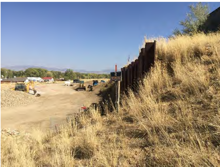
Photo #3: Materials stockpiled against the highwall on the south side of the LMO boundary. The stockpiled material has decreased in volume. Photo taken September 24, 2020.
