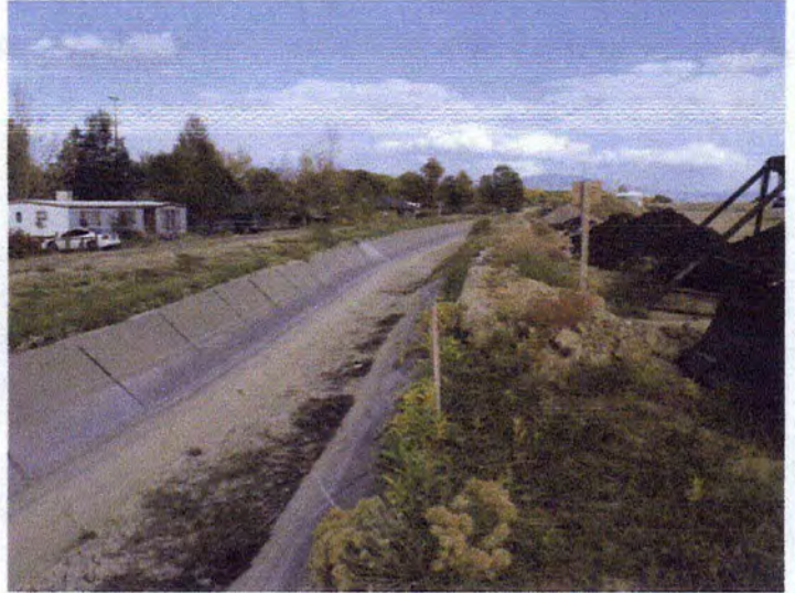
Photo #2: General overview of constructed berm and canal looking east. Sediment continues to deposit in canal.
