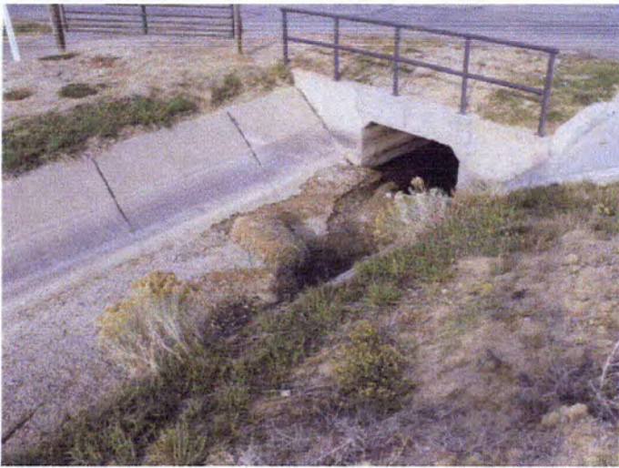
Photo #3: General overview of canal looking northeast direction. Sediment control measures (hay bale) located in the canal.
