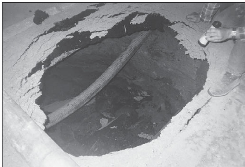
Fig 2.2.2 Subsidence hole (Crowell 2010)
