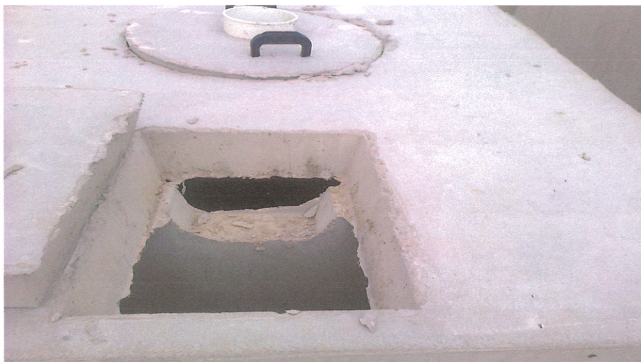
Wind River Model 1000 Tank with cast inlet baffle and cutout for gas venting.
